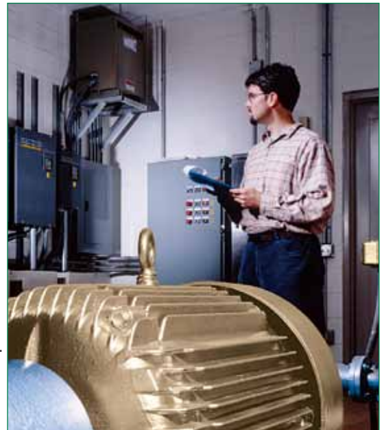
A Baldor Super-E motor and Inverter Control provide premium energy efficiency and improved process control to a municipal water treatment facility.
